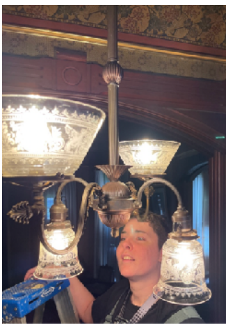
Miranda is installing the fixture in the middle hallway. We can now see the ceiling and wall papers. Beautiful
